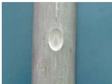
b) Corroded Pipes
