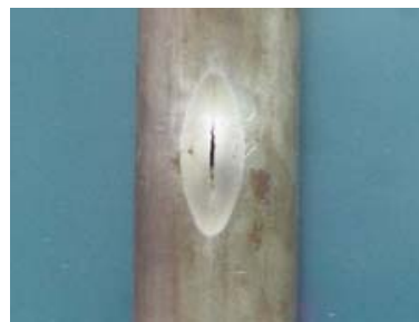
c) Corroded Pipes
